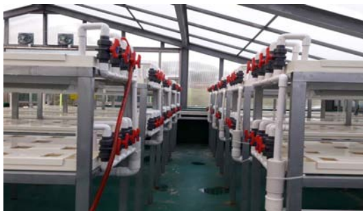
Influent water line
